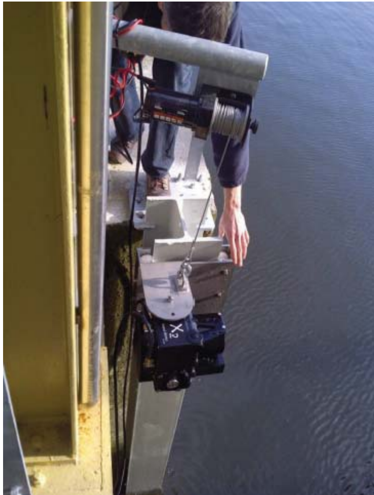
Figure 3 Mounting at Arzal dam, France
